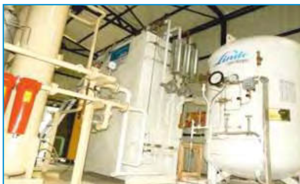
Liquid N2 Plant
